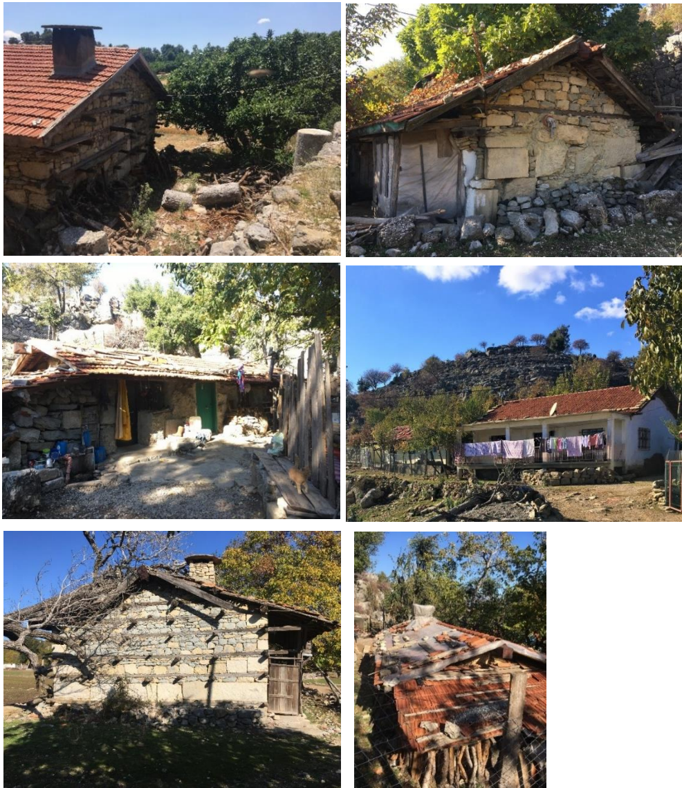
Figure 3.60: The bad and good conditions of the traditional houses in Altinkaya, and new house, author, 2021.
